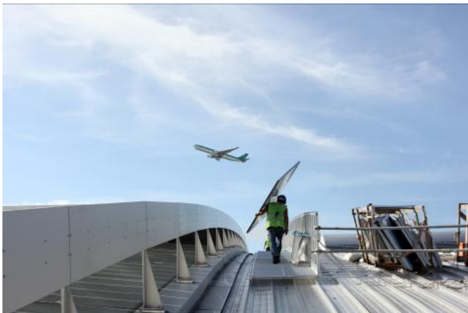
View of a construction worker carrying an external cladding panel across the roof of the new Terminal. The cladding and glazing contract for T2 is being delivered by the Portuguese firm, Martifer.
