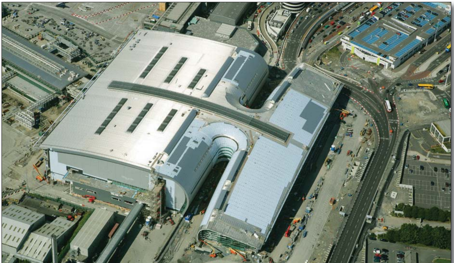
The much awaited Terminal Two at Dublin Airport is nearing completion and is expected to come into operation in November 2010. While unfortunate that it will open at a time of depressed traffic volumes, T2 is a critically important piece of national infrastructure that will serve Dublin and Ireland well for several decades to come.
